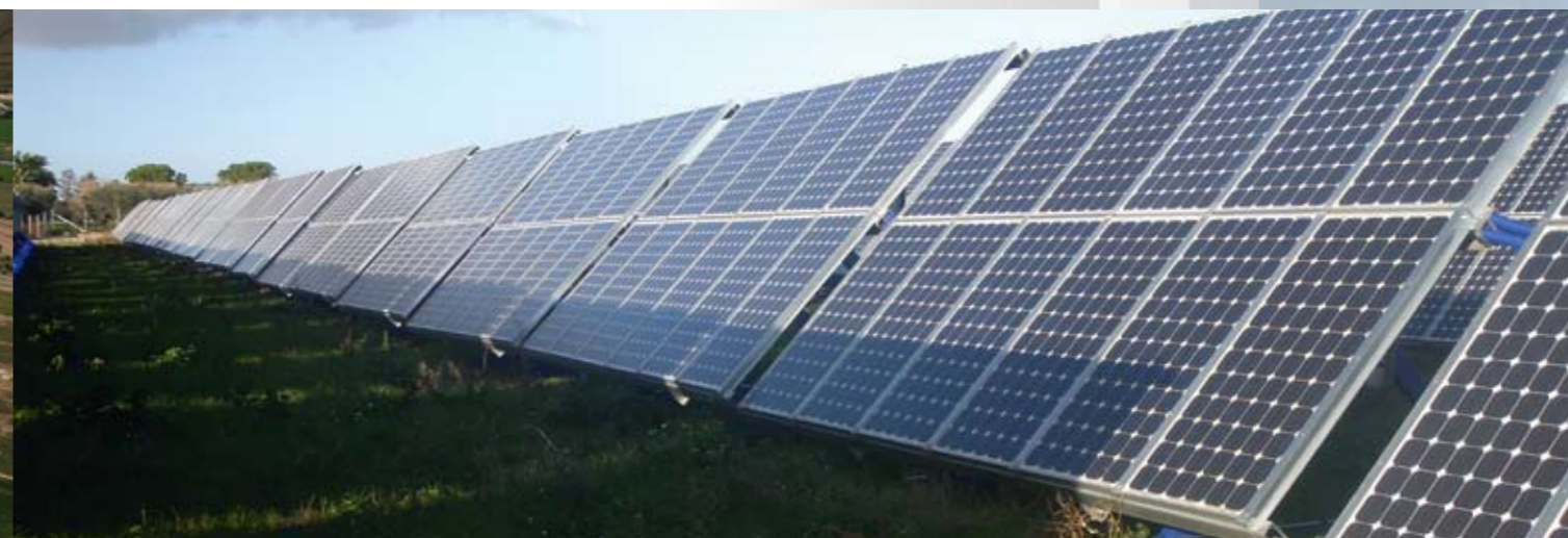
PV project using CSUN modules in Puglia, 4.3 MW
