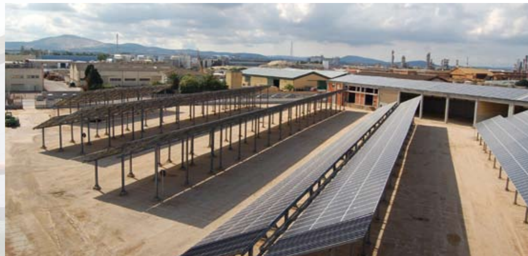
BIPV project using CSUN modules in Serdegna, 1.5 MW
