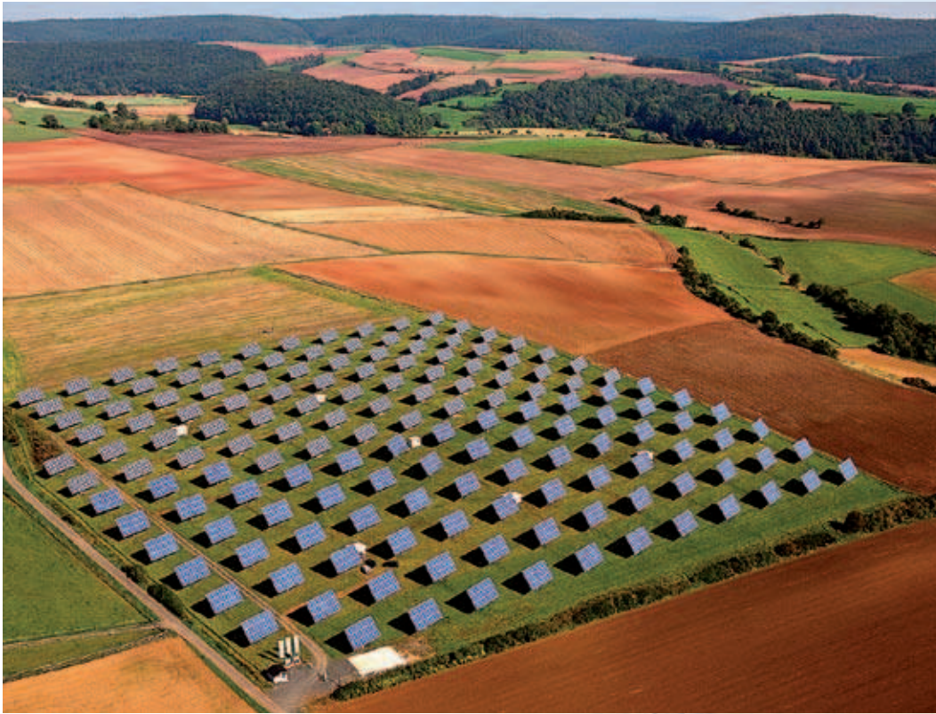
In 2008, ConSolaris installed 151 solar trees on the outskirts of Edertal.
